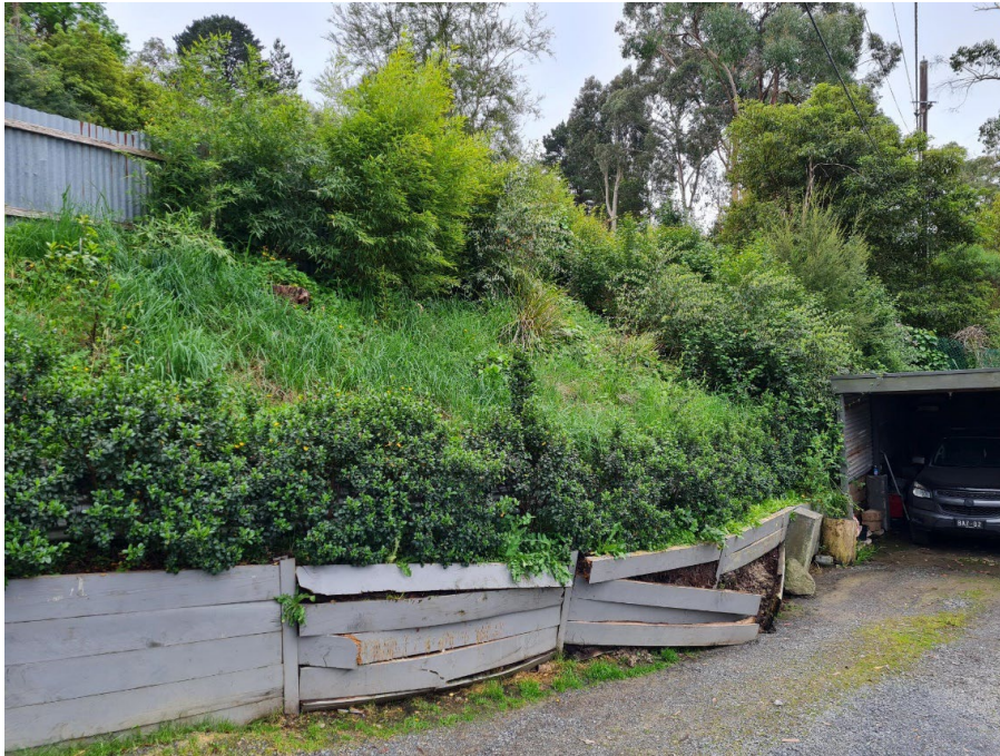
Figure 2 Landslip at Mount Evelyn on 5 October 2023
